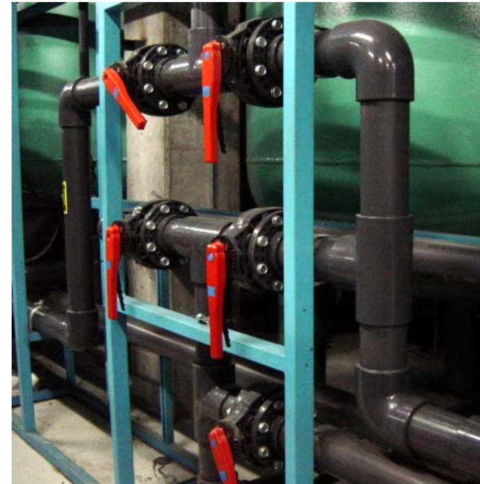
Industrial water treatment
